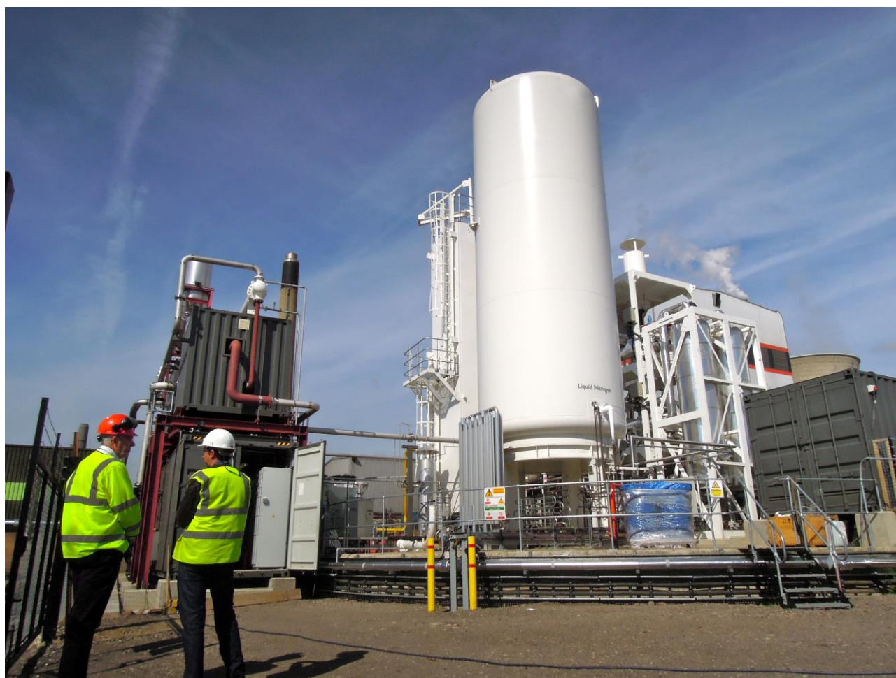
Figure 2 The 350 kW Highview Power Storage pilot plant in Slough, UK (reprinted courtesy of Highview Power Storage)
